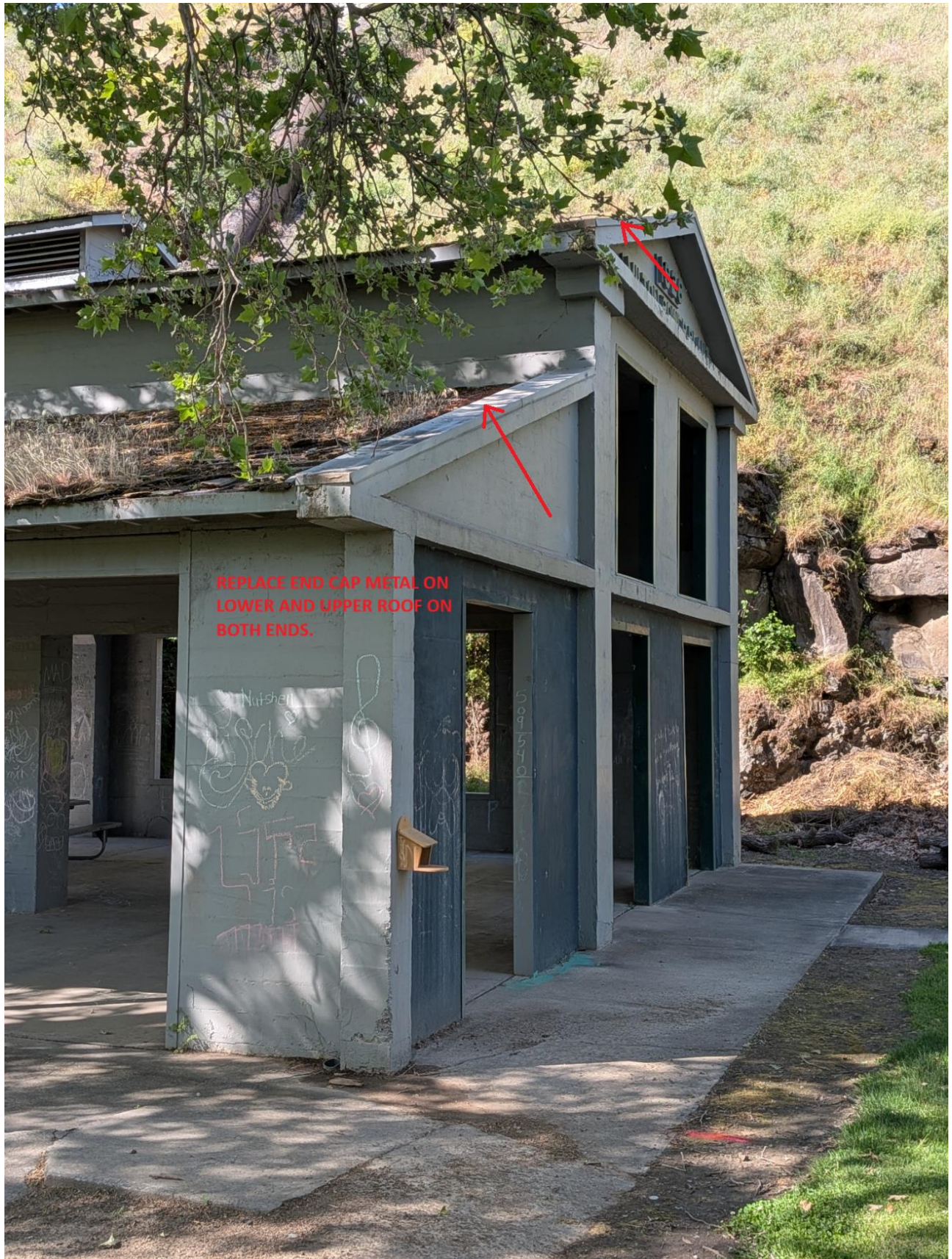
Figure 1 - Marie Dorian Park Power Plant Shelter showing the location of the metal end caps that need to be replaced.
