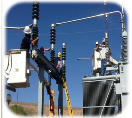
City Journeymen Linemen performing substation maintenance (left to right) – Rick Duede, Richard Jolly, Scott Graff & Shannon Brownie. Not pictured but also on job – Rich Gannon and Bill Daugherty.
