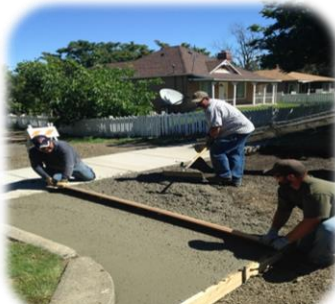
Public Works employees replacing alley approach (left to right) – Emilio Sandoval, Shane Wright & Levi Nored. Not pictured but also on the job – Dave Robertson & Dan Verkist
