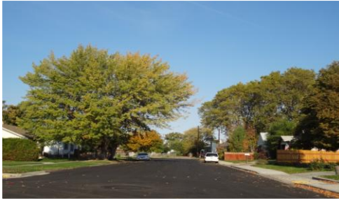
S. Mill Street Widening Improvements Photo submitted by: Jeremy Morris, P.E., Anderson-Perry & Associates, Inc.
